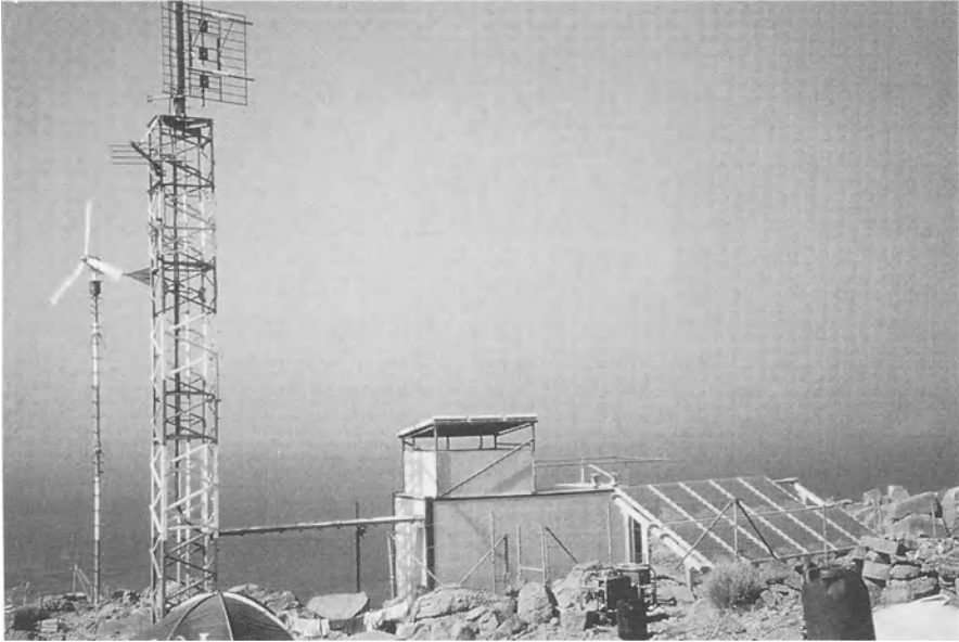
Fig. 1.10. Wind-generator installation and solar generator of a mains-independent hybrid power supply system (photo by courtesy of Siemens AG)
