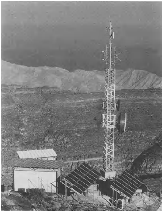
Fig. 16.12. Solar generator of a mains-independent power supply system. (Photo by courtesy of Siemens AG)
